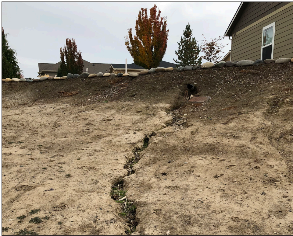
Problem Area #1 - Hillside erosion at the end of 3rd Avenue.
